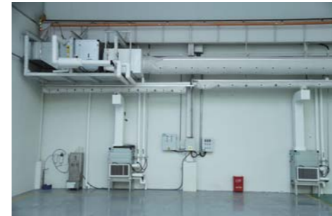
Air conditioning in workshop 5°C - 12°C
