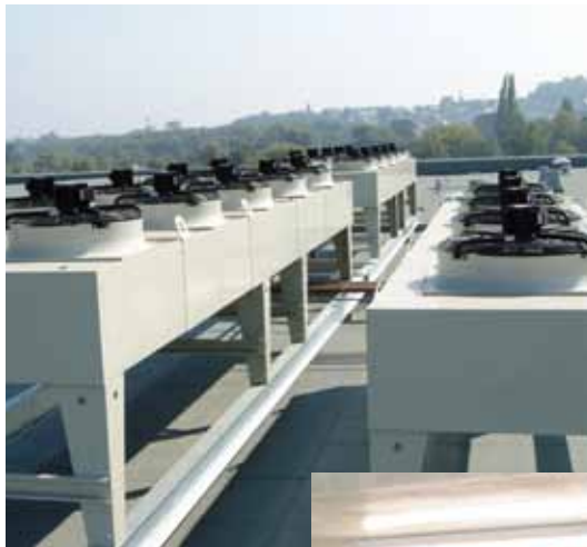
Air conditioning application
